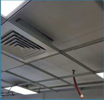
T-Grid suspended Ceiling
